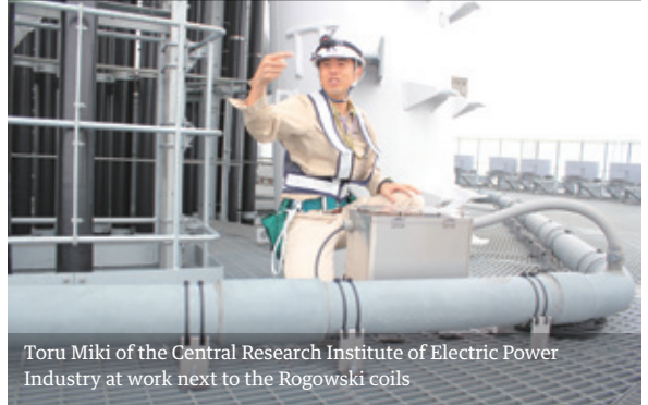
Rogowski coils installed to enclose steel poles at a point on the Tokyo Skytree 497 meters above the ground
