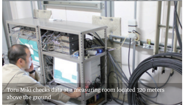
Toru Miki of the Central Research Institute of Electric Power Industry at work next to the Rogowski coils
